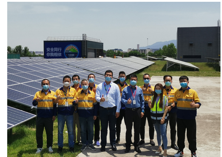
The Xi'an site team after completing the second phase of photovoltaic (PV) panel installation.
